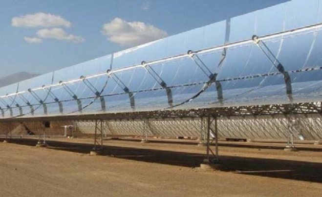
Parabolic Trough system at Andasol 1, Spain
